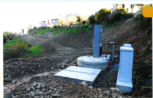
Station de relevage
